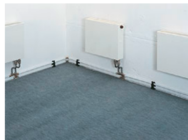
Radiator connection from the skirting board
