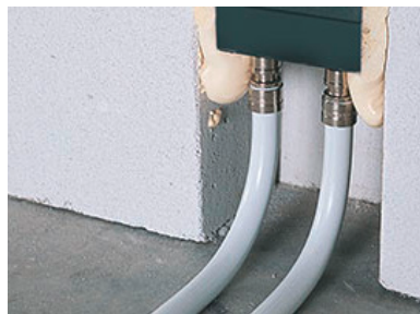
Radiator connection from the wall
